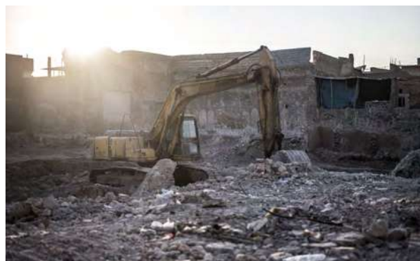
A mechanical shovel in the middle of the ruins of an old house in Mosul, contaminated by explosive ordnance. © F.Vergnes / HI
