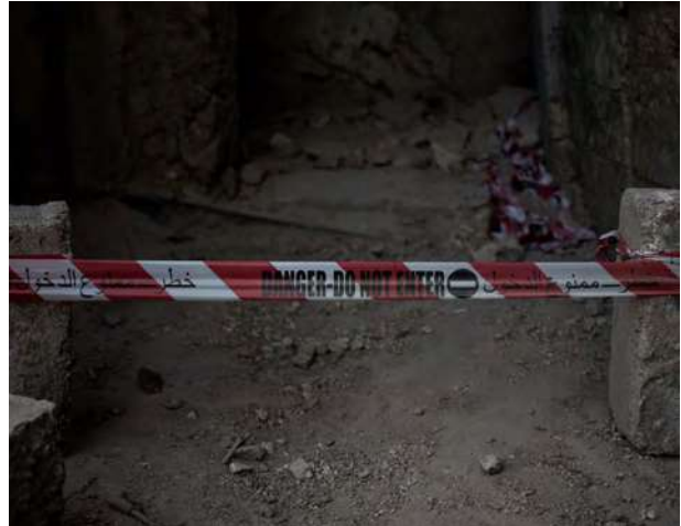
A danger warning at the entrance of a contaminated house in Mosul. © F.Vergnes / HI
