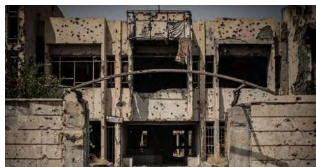
A destroyed health center in Mosul. © F.Vergnes / HI
